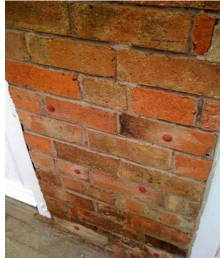
Studs are only visible sign of flood defences
